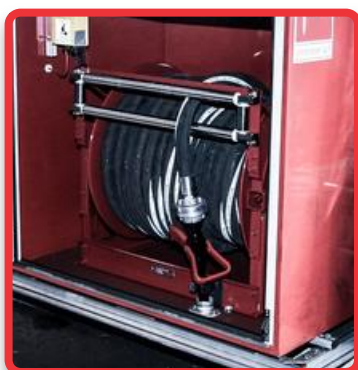
One Seven Wall Hydrant
